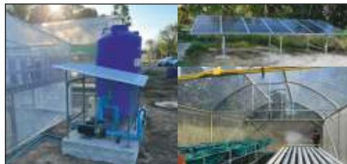
MODEL : 1800 WATT, DISCHARGE : 145'000 LPD (THAILAND)
